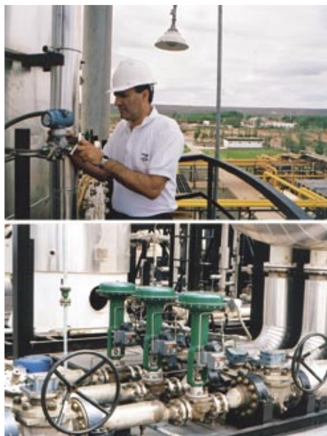
FIG. 3 Intelligent instruments such as those communicating via FOUNDATION fieldbus in the LTS 2 plant form the field base of the digital plant architecture. (Above: differential pressure transmitter. Below: digital valve controllers on control valves.)
